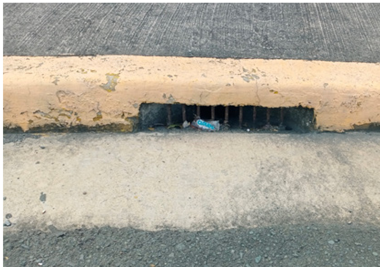
Figure 48. Storm Drain near Passenger Terminal Collection Point last September 25, 2021
