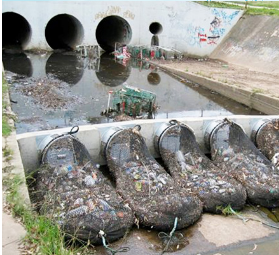
Figure 45. StormXTM Storm Water Runoff Trash Traps (Storm Water Systems, 2020)
